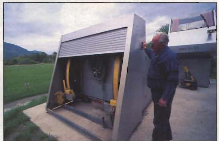
Two of the cable drums and, behind, the control room.
